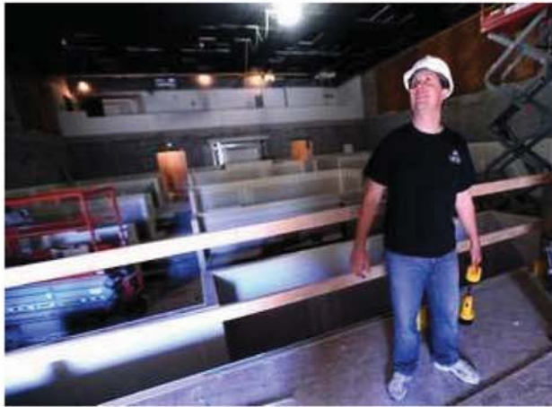
Purchase this Photo Kurt Terrio, owner and producer of Carousel Dinner Theatre, stands on the stage of the theater's new location at 3750 S. Mason St., in Fort Collins. Formerly the Mann 4 Movie Theater, the Midtown Arts Center will be completed and host its first musical, 'White Christmas' on Nov. 19. The center's dinner theater will seat 260 people. (Dawn Madura/The Coloradoan)
